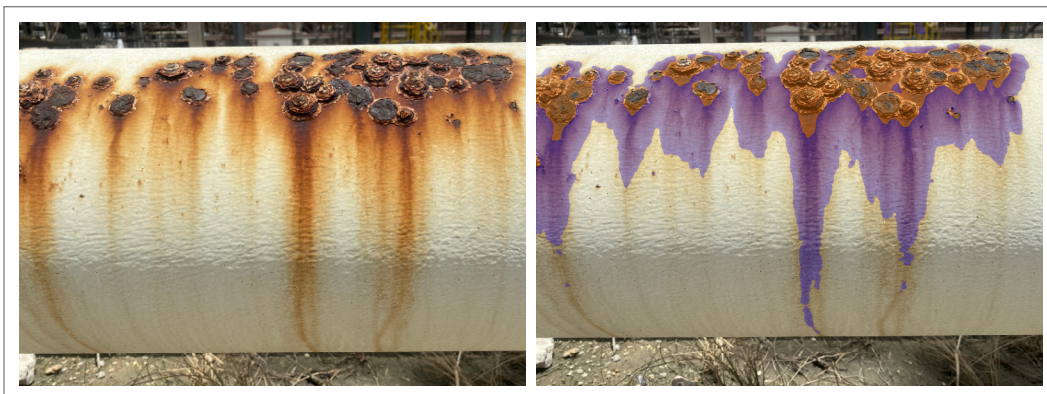
Corrosion Segmentation Results
